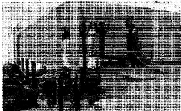
Owners of homes in danger of imminent collapse due to erosion could receive assistance under the NFIP to demolish or relocate their homes.
